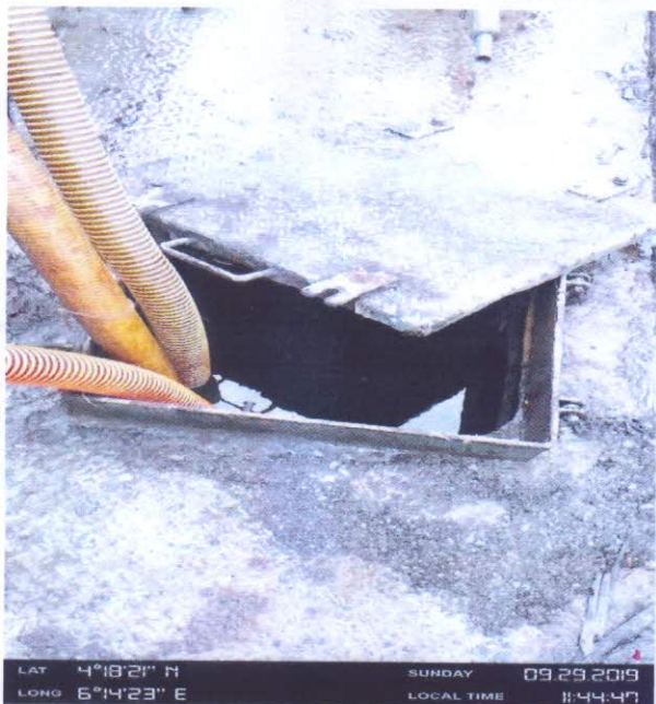
SPILL POINT ON ARRIVAL.
